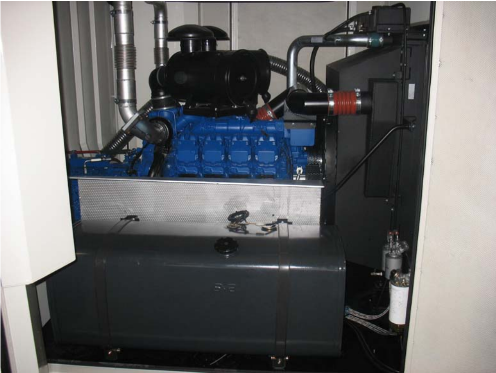
Deutz engine and fuel tank
